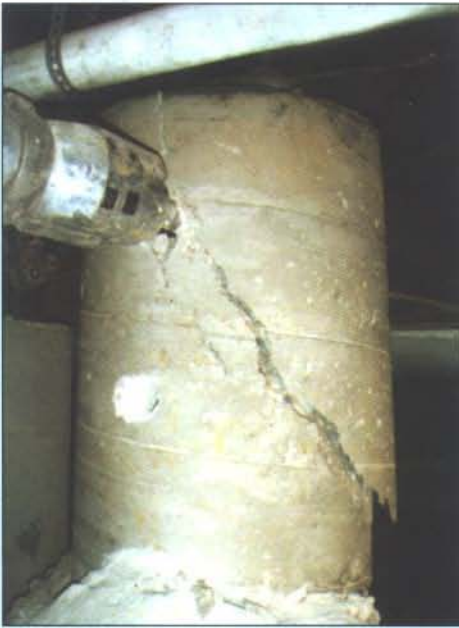
Spreader bar breaking existing pier.
